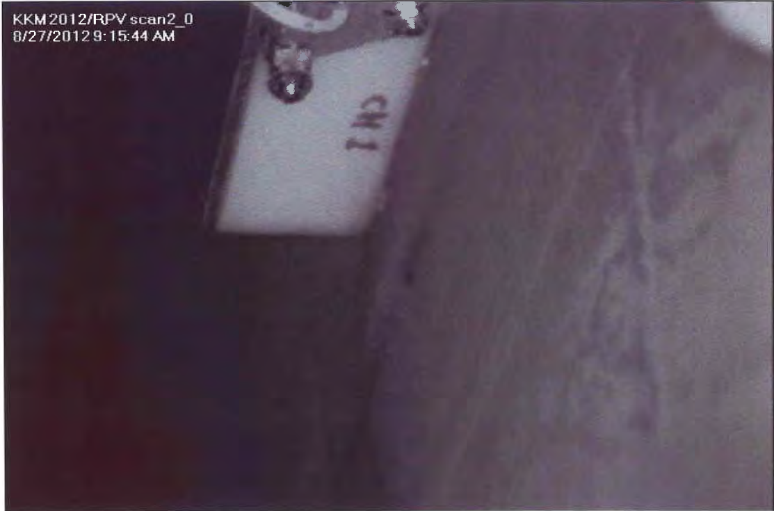
Vertical Clad Patch Seen in Patches 10 and 11
